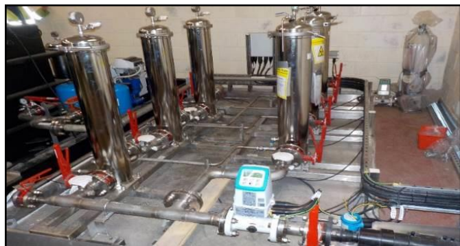
New Effluent Treatment plant within the Low-Level Waste Transfer Facility.
