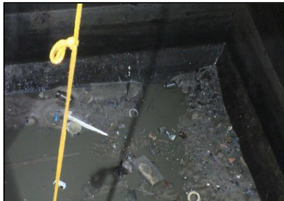
Residual sludge and miscellaneous debris in Sludge Retention Tank 3 in WILWREP
