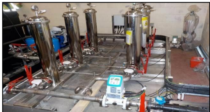
New Effluent Treatment plant within the Low-Level Waste Transfer Facility.
