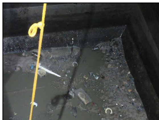
Residual sludge and miscellaneous debris in Sludge Retention Tank 3 in WILWREP
