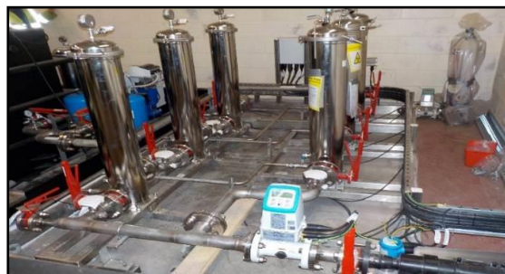
Picture above of New Effluent Treatment plant within the Low-Level Waste Transfer Facility
