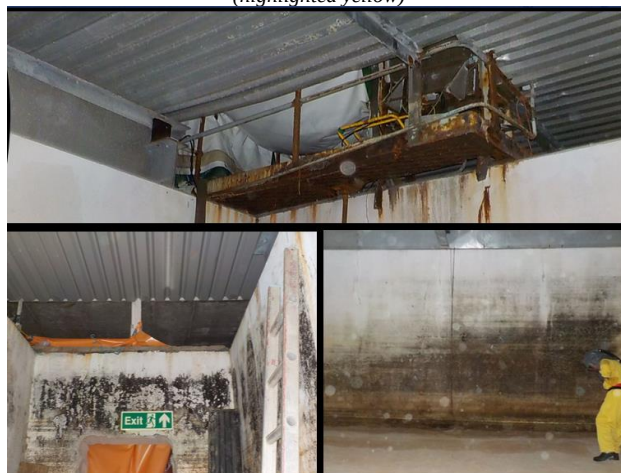
Internal views of Delay tanks
