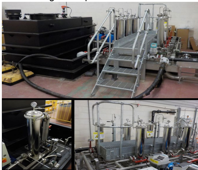
New Effluent Treatment plant within the Low-Level Waste Transfer Facility.
