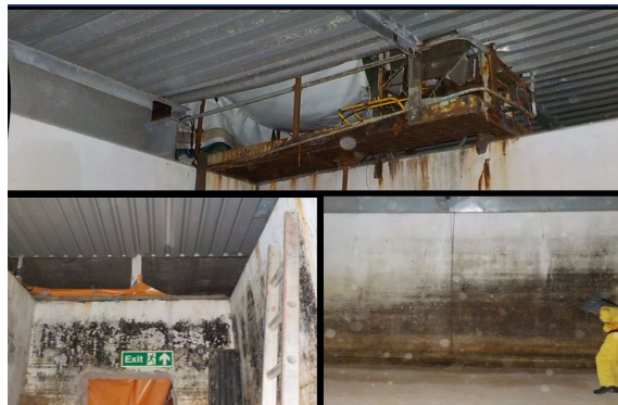
Internal photos of Delay Tanks
