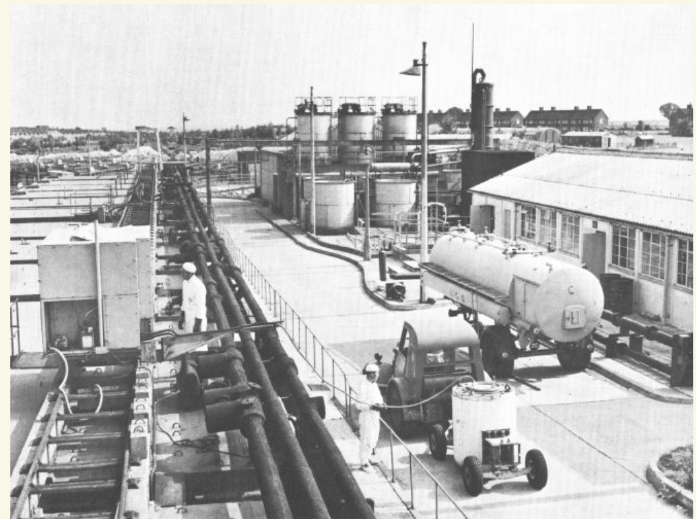
FIG. 8. MOBILE RECEIVER ON HIGH LEVEL STORAGE TANKS
