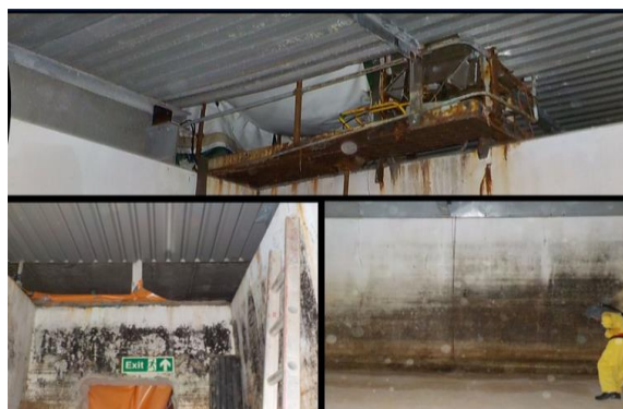
Internal photos of Delay Tanks
