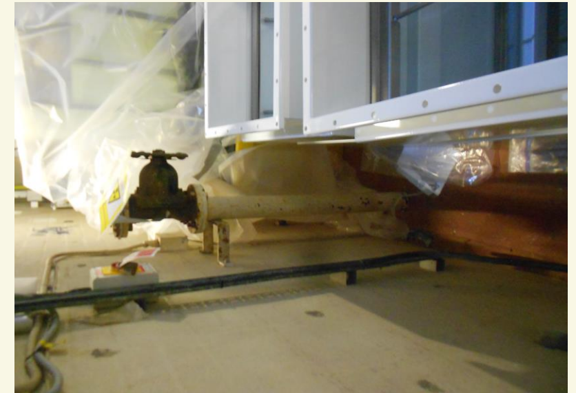
Redundant pipework and valves
