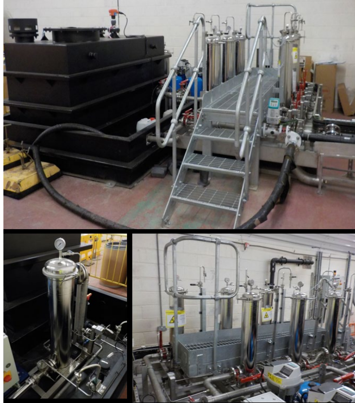
New Effluent Treatment plant within the Low-Level Waste Transfer Facility
