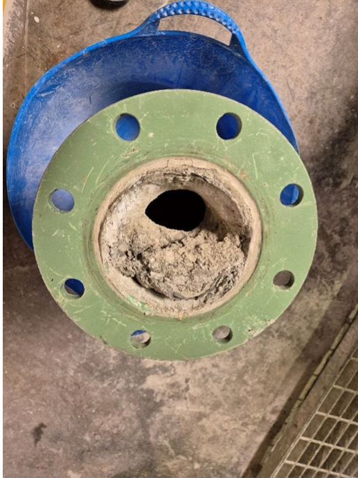
Before – powder delivery pipe restricted
